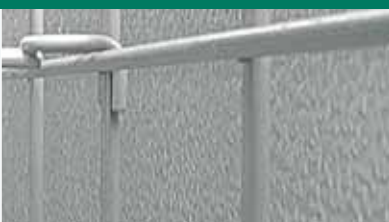
3.) Frost-free inner wall after the defrosting process
